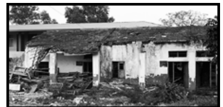
Derelict Building in School Area
