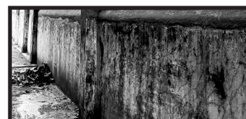
Old Low Moldy School Wall
