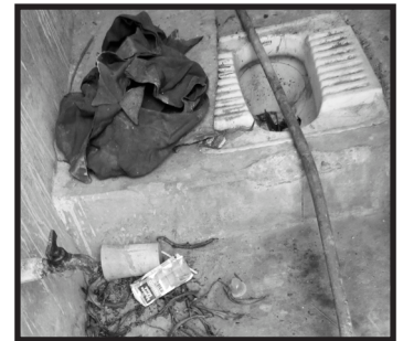
Dead toilet at School
