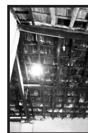
Leaky Roof Over Beds
